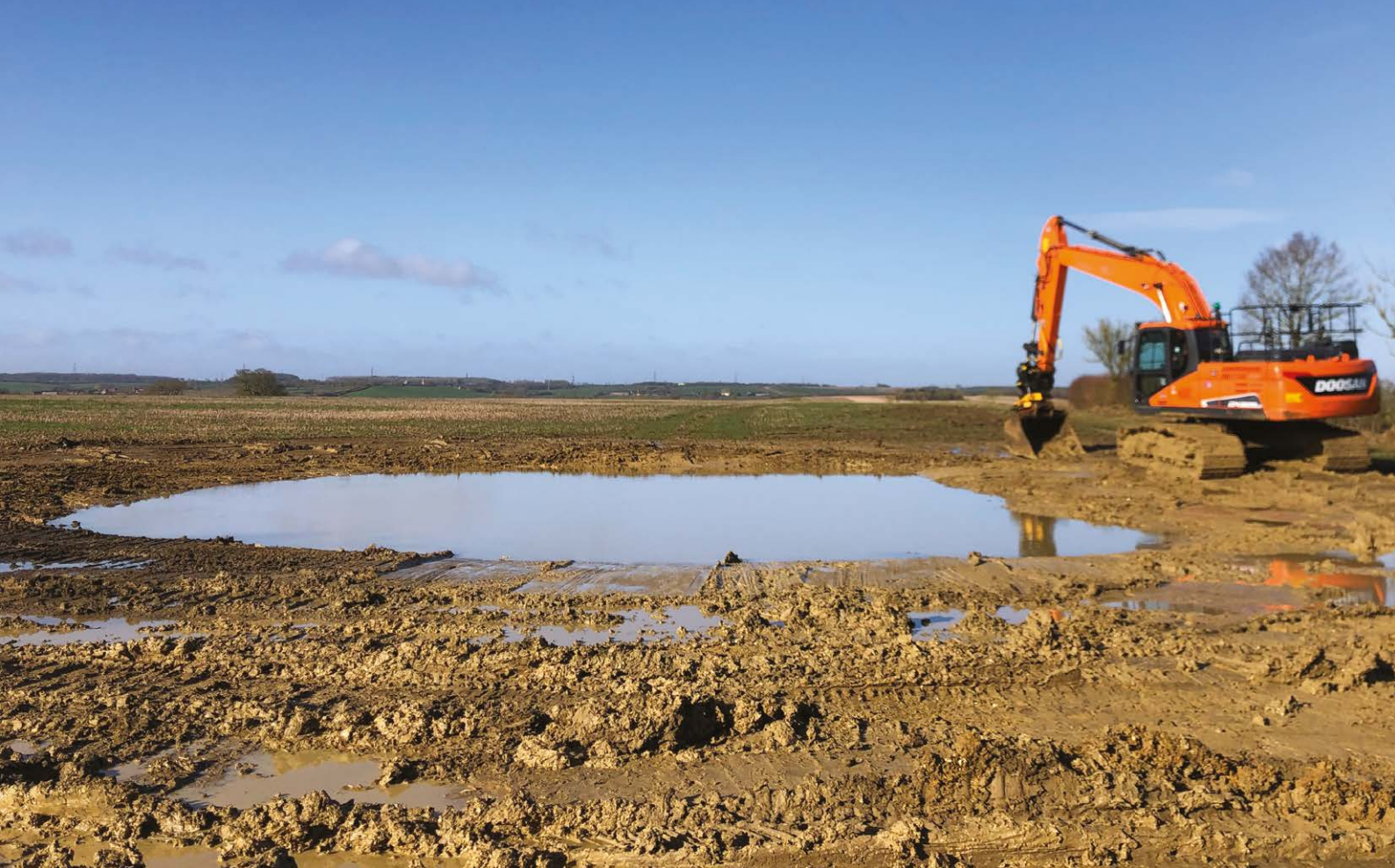
Fig. 29. Pond creation in progress at Boothby Wildland in February 2023. We like to keep digger track marks – see foreground – in and around our ponds as this creates microhabitats for all sorts of wildlife. We leave the finishing to weathering by rain, wind and frost, so our ponds eventually have a more natural look.
