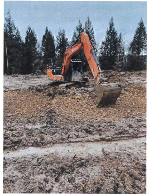
Early stages in the construction of a Great Crested Newt District Licensing Scheme pond creation project at Nagshead Plantation, Forest of Dean
