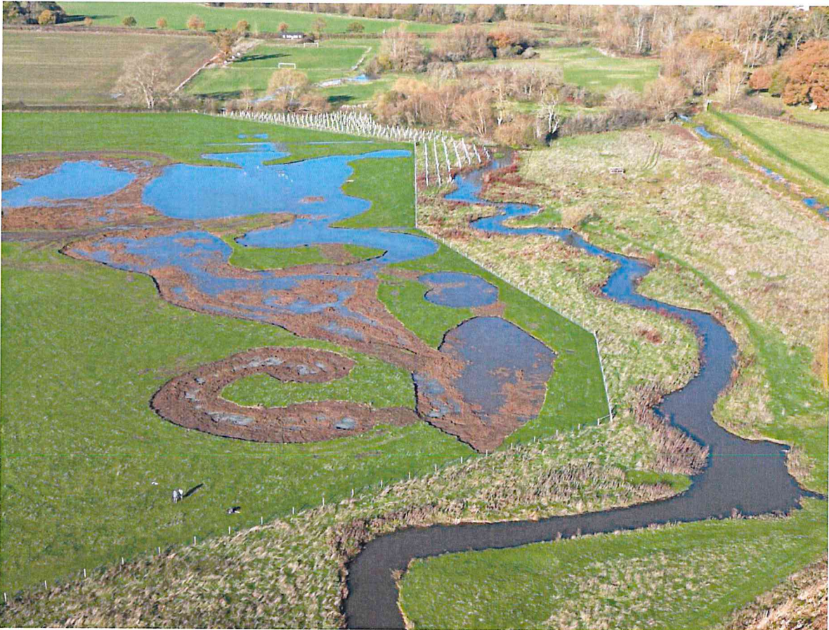
Fig 2. In 2022-23 we completed the first stages of Building the Oxfordshire Freshwater Network, funded by the Government's Green Recovery Challenge Fund. The picture shows the creation of new floodplain wetland mosaic habitat at the National Trust Buscot and Coleshill Estate on the Oxfordshire-Wiltshire border. On this site we are addressing one of our core aims which is to focus on the restoration of Historic Floodplains, a key component of the Freshwater Network. This is the floodplain of the R. Cole where we first started practically assessing the benefits of river restoration in the mid-1990s, creating the sinuous river channel shown in the picture as part of an EU LIFE funded demonstration project.
