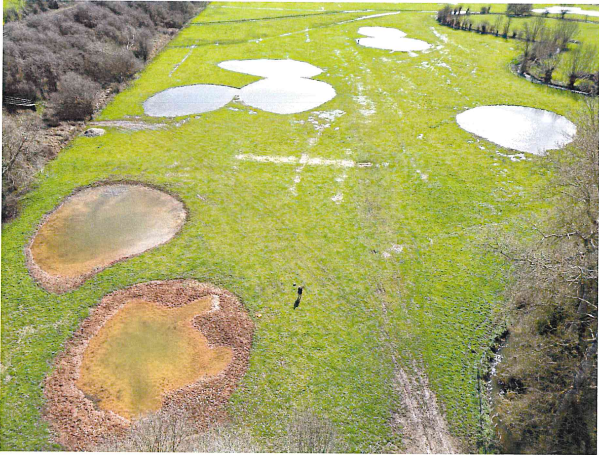
Fig 1. In 2022-23 we completed the first stages of Building the Oxfordshire Freshwater Network, funded by the Government's Green Recovery Challenge Fund. The picture shows the creation of new floodplain wetland mosaic habitat at Manor Farm in Buckinghamshire continuing our work to build the Freshwater Network in this area. On this site we are addressing one of our core aims which is to focus on the restoration of Historic Floodplains, a key component of the Freshwater Network. This is the floodplain of the R. Thame (the river itself is just out of view at top of the picture) and shows ponds in the winter of 2022-23. As water levels drop in the summer, the waterbodies that are linked in this winter picture (top left, top right) will separate out to form ponds and pools of varying sizes and depths, an approach which our work has shown maximises the variety of freshwater species on a site. Green Recovery Challenge Fund support also contributed to the creation of the Freshwater Network in the New Forest.
