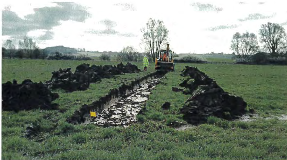
Digging trial archaeological trenches in preparation for the construction of a wetland complex on the Waddesdon Estate in Buckinghamshire, part of our catchment management work with the River Thames Conservation Trust.
